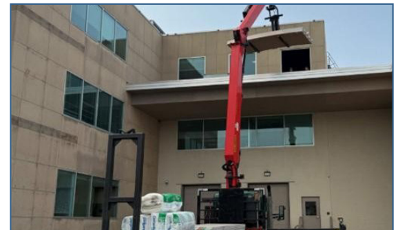
CRANE HOISTING SHEETROCK TO THE 3RD FLOOR WINDOWS FOR THE LIFE COMPANY'S SPACE EXPANSION
